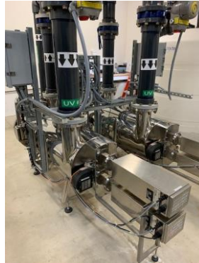
WTP UV System
