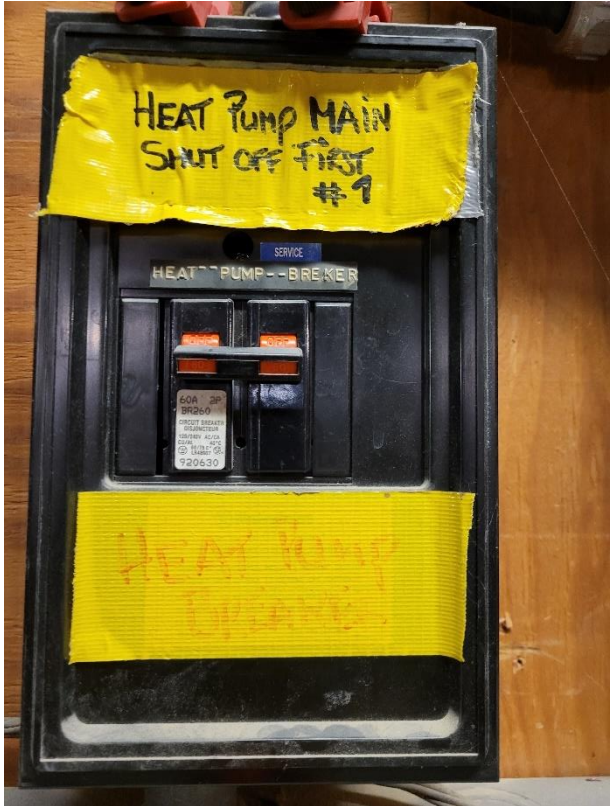
Image 8: Existing electrical breaker
