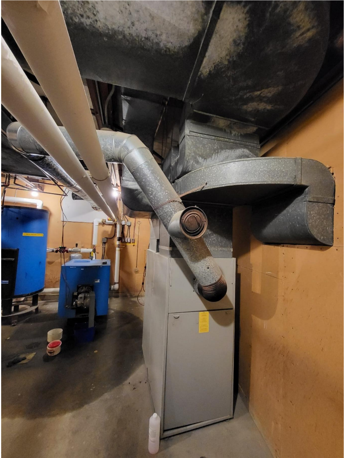
Image 5: Diesel furnace and ductwork
