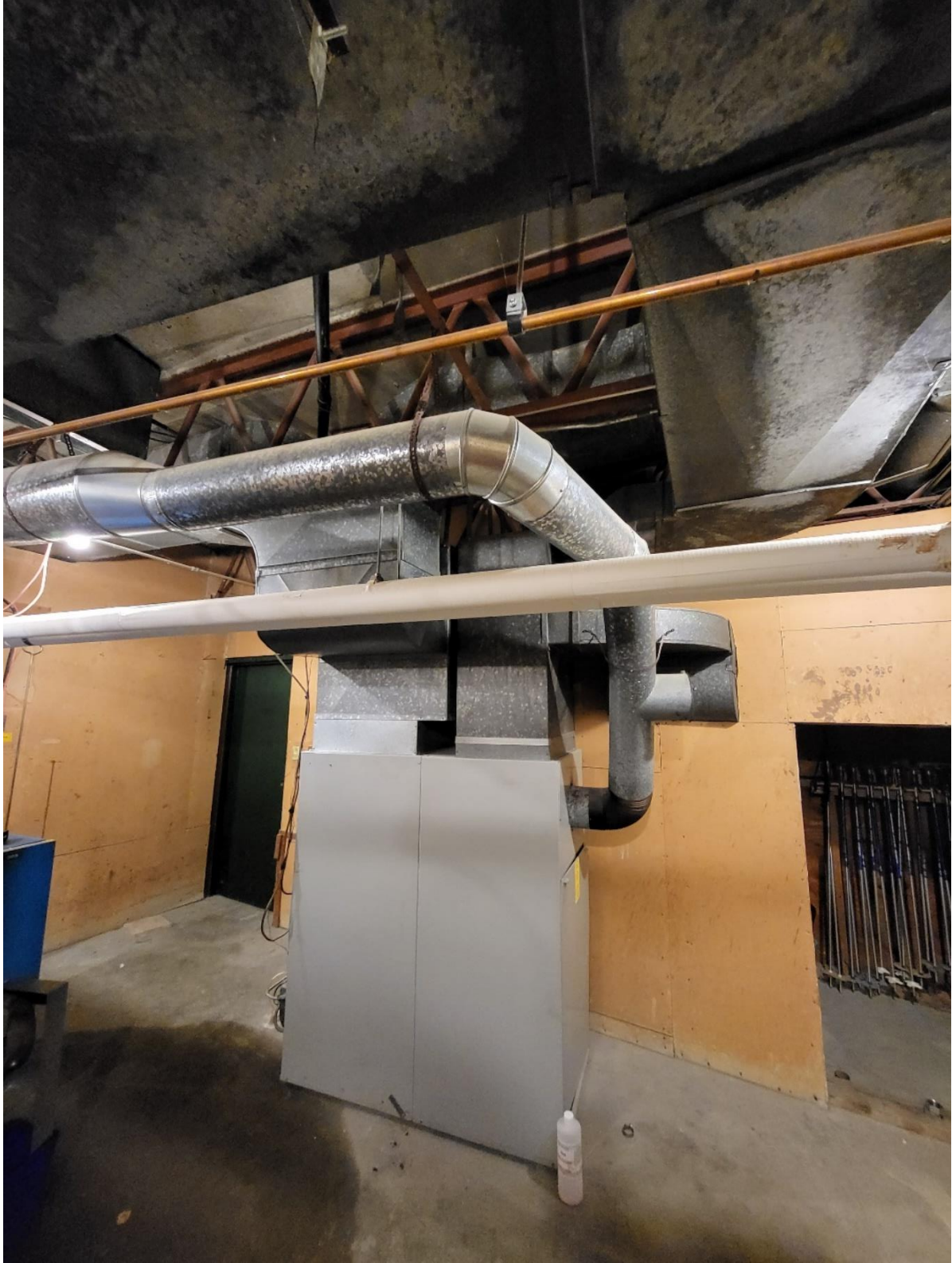
Image 6: Diesel furnace and ductwork
