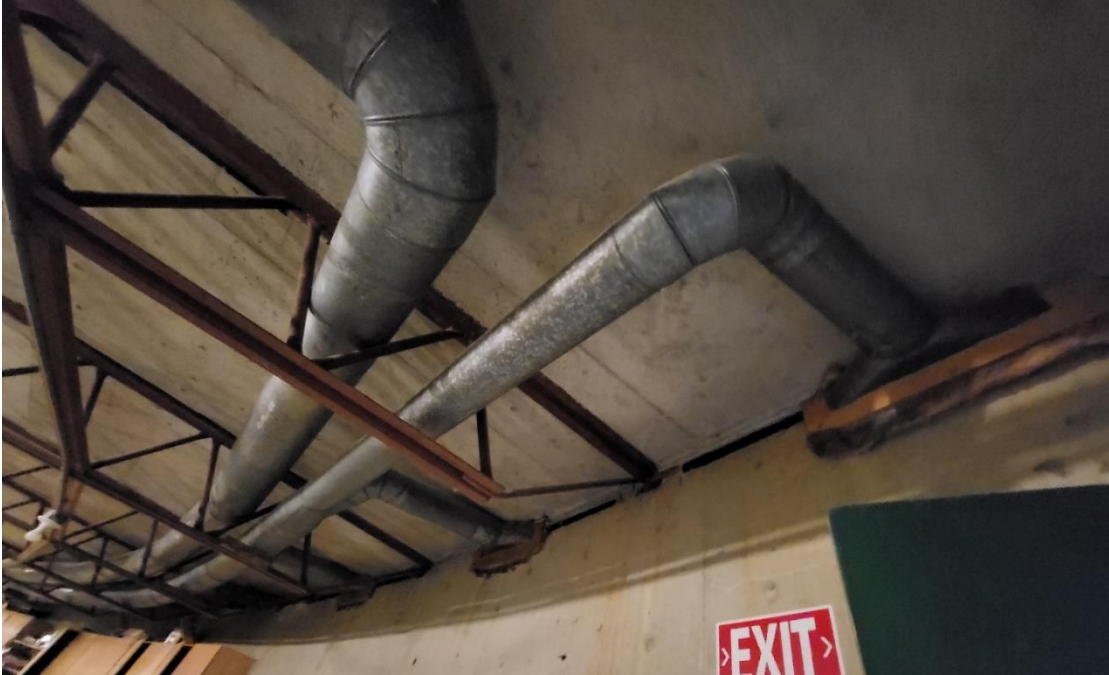
Image 18: End of ductwork in area "B"
