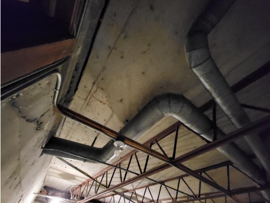
Image 17: End of ductwork in area "B"
