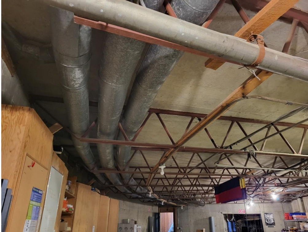
Image 15: Ductwork in area "B"
