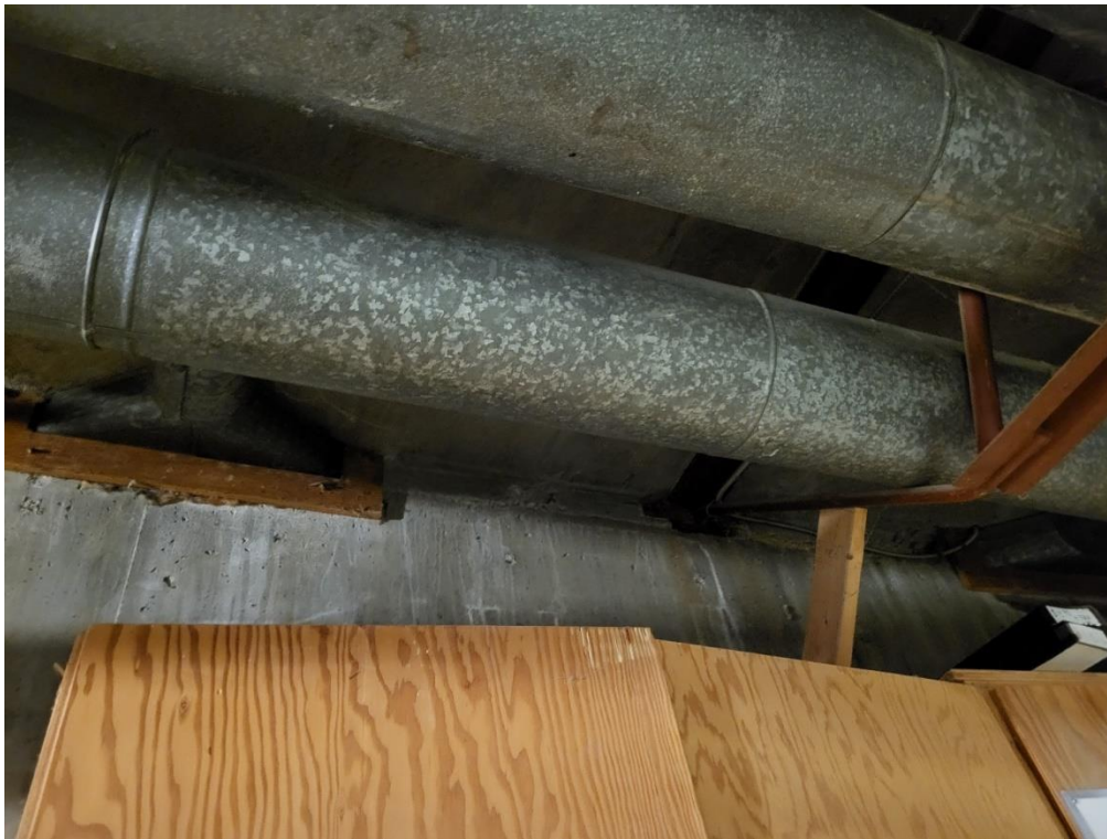
Image 16: Ductwork in area "B", last vent of one run
