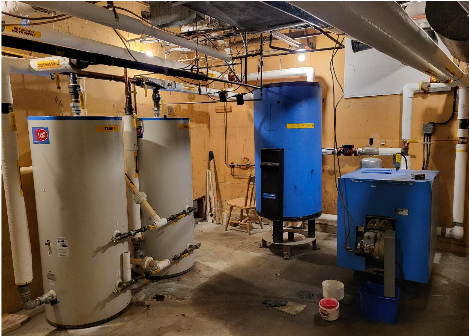
Image 1: Heat exchange tanks, storage tank, and boiler.
